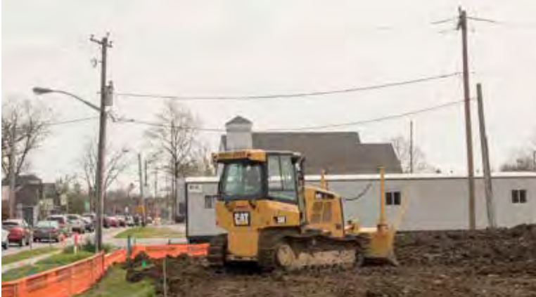
Pictured Above The actual ground breaking, looking south towards US 136 (Main Street) west side of street, the former St. Malachy property.
